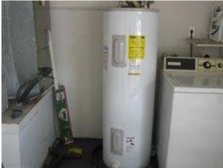
Photo 12 Water heater in garage
