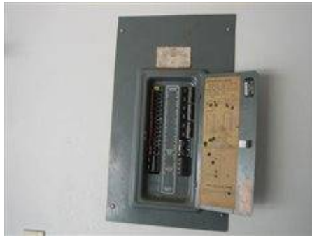
Photo 15 Main electric panel in garage
