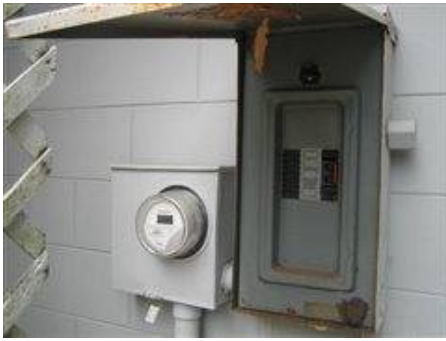
Photo 8 Exterior electric service panel into house
