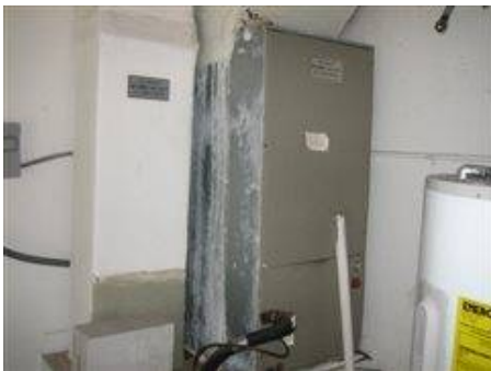
Photo 14 Air Handler in garage
