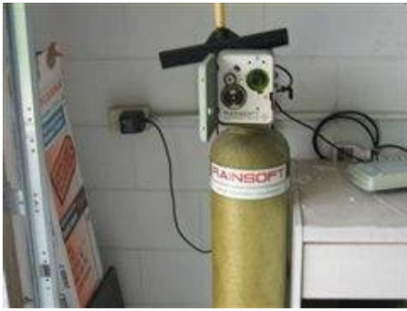
Photo 10 Water conditioning system
