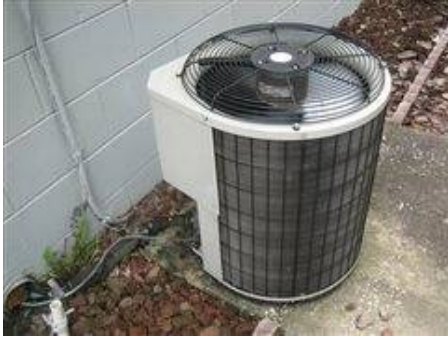
Photo 6 Heat Pump Compressor
