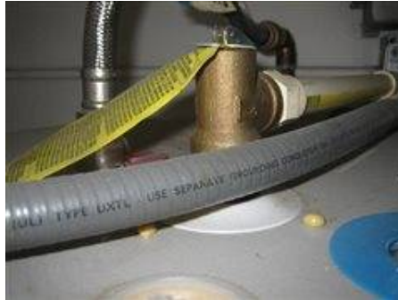
Photo 13 Water heater Temperature Pressure Relief Valve
