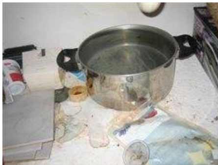
Photo 30 Under leaking trap in master bath sink was a pot full of water from continual long-term leaking
